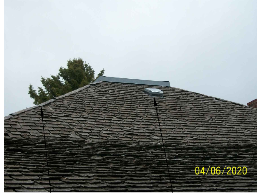
REMOVE & REUSE EXIST. METAL RIDGE CAPS EX. STATIC VENTS TO REMAIN IN-PLACE
