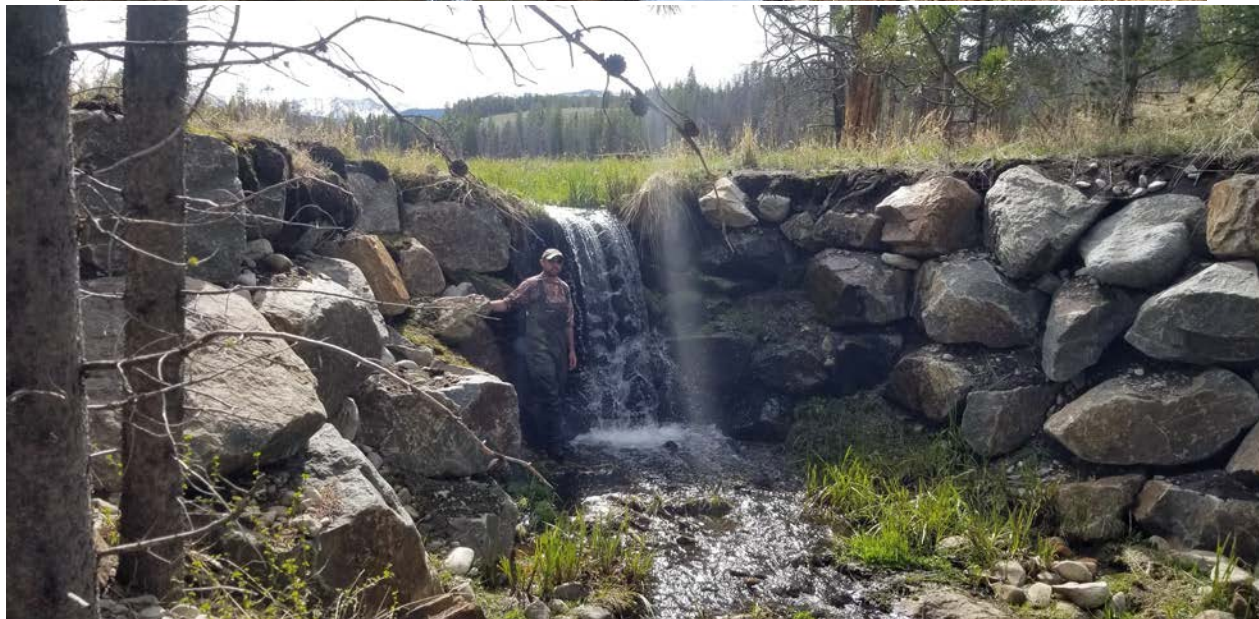
Figure 4. Fish barrier on the outlet of Van Houten Lake. Photo on top is immediately after construction in the fall of 2015 and the figure on the right is 6 years after construction in 2021.
