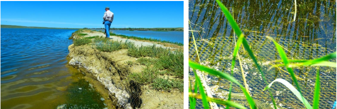
Figure 7: Erosion on the DU (1988) dike and the flooded water control structure
