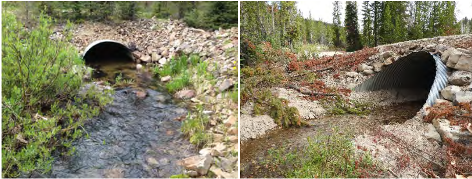
FIGURE 16. MONARCH CREEK CULVERT REPLACEMENT BEFORE (L) AND AFTER (R). PHOTOS COURTESY OF THE US FOREST SERVICE AND FWP.
