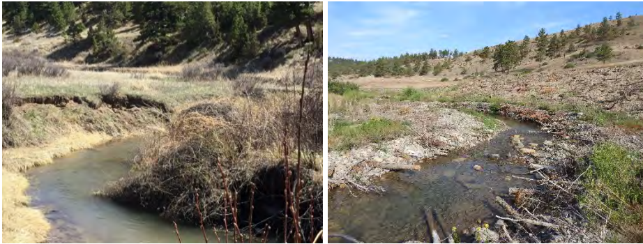
FIGURE 7. BEAVER CREEK CHANNEL RECONSTRUCTION BEFORE (L) AND AFTER (R) CONSTRUCTION. PHOTOS COURTESY OF THE US FOREST SERVICE AND FWP.
