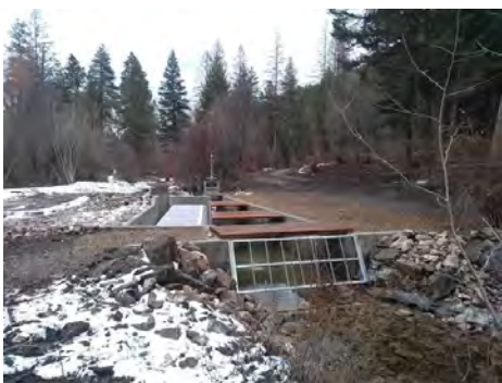
FIGURE 14. LOLO DITCH FISH SCREEN AFTER COMPLETION. PHOTO COURTESY OF THE CLARK FORK COALITION.
