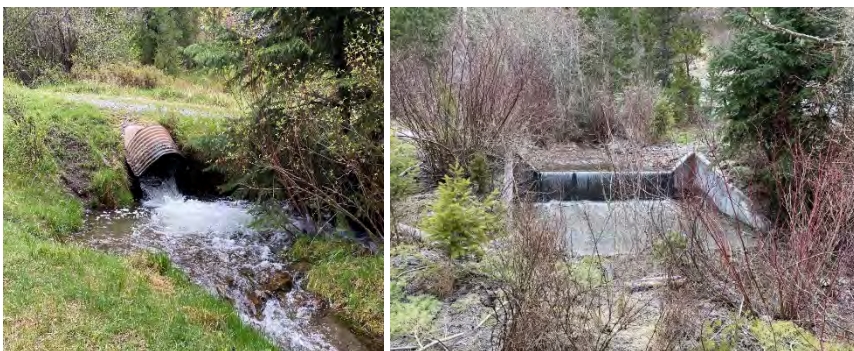
FIGURE 5. LITTLE PARK CREEK BARRIER BEFORE (L) AND AFTER (R) CONSTRUCTION. PHOTOS COURTESY OF THE CLARK FORK COALITION.
