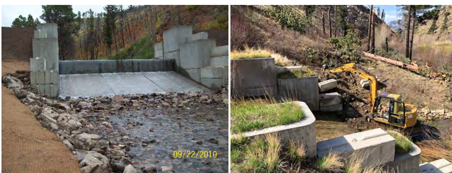
FIGURE 22. THE COTTONWOOD CREEK BARRIER AFTER CONSTRUCTION (2010, L) AND AS IT WAS REPAIRED IN 2021 (R).
