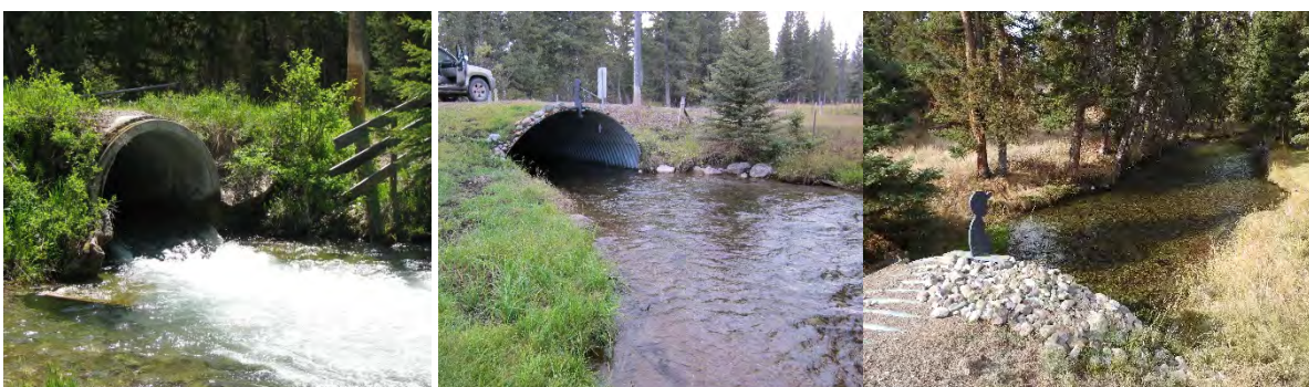
FIGURE 26. LINCOLN SPRING CREEK BEFORE (L) AND AFTER (MIDDLE) CONSTRUCTION, AND IN 2021 (R).
