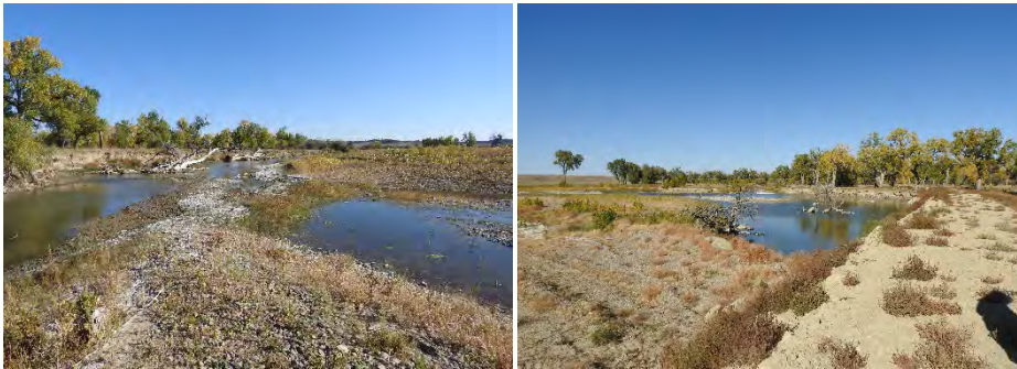
FIGURE 17. MUSSELSHELL RIVER MCCLEARY CHANNEL RESTORATION AFTER CONSTRUCTION, WHERE THE AVULSION OCCURED (L) AND CHANNEL PLUG (R).
