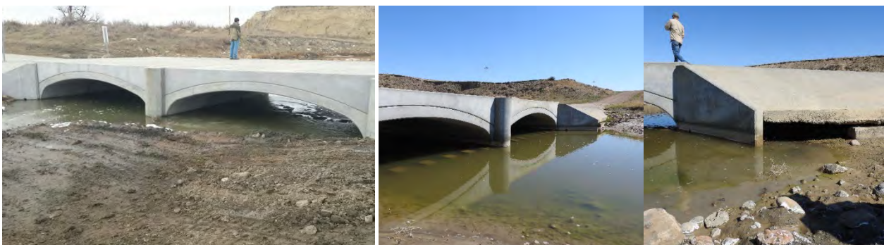
FIGURE 38. THE REDWATER RIVER NICKWALL CROSSING AFTER CONSTRUCTION (2016, L) AND IN 2021 (MIDDLE, R). NOTE THE EROSION OF THE WINGWALL TO BE REPAIRED IN 2021 (R).
