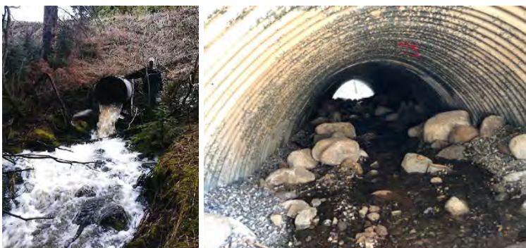
FIGURE 11. EAGLE CREEK CULVERT REPLACEMENT BEFORE (L) AND AFTER (R) CONSTRUCTION. PHOTOS COURTESY OF THE US FOREST SERVICE AND FWP.
