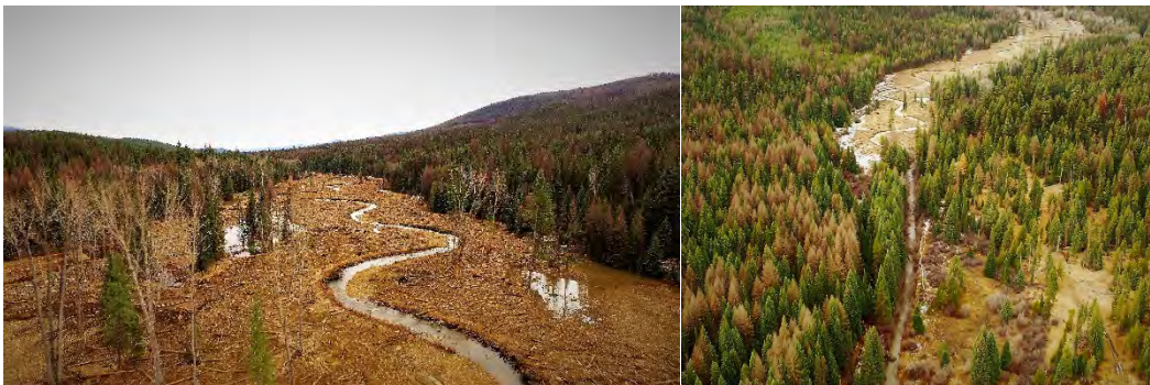
FIGURE 18. NINEMILE CREEK AFTER CONSTRUCTION, SHOWING THE FINISHED CHANNEL AND FLOODPLAIN (L) AND THE CONTRAST BETWEEN UPSTREAM COMPLETED AND DOWNSTREAM PROPOSED WORK (R).
