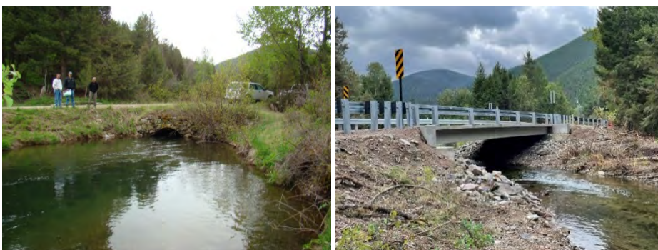
FIGURE 3. POORMAN CREEK CULVERT REPLACEMENT BEFORE (L) AND AFTER (R) CONSTRUCTION. PHOTOS COURTESY OF THE BIG BLACKFOOT CHAPTER OF TROUT UNLIMITED.
