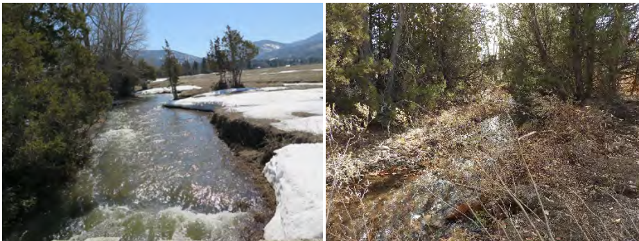
FIGURE 19. POORMAN CREEK BEFORE (L) AND AFTER (R) CONSTRUCTION. PHOTOS COURTESY OF BIG BLACKFOOT CHAPTER OF TROUT UNLIMITED AND FWP.FIGURE 19.
