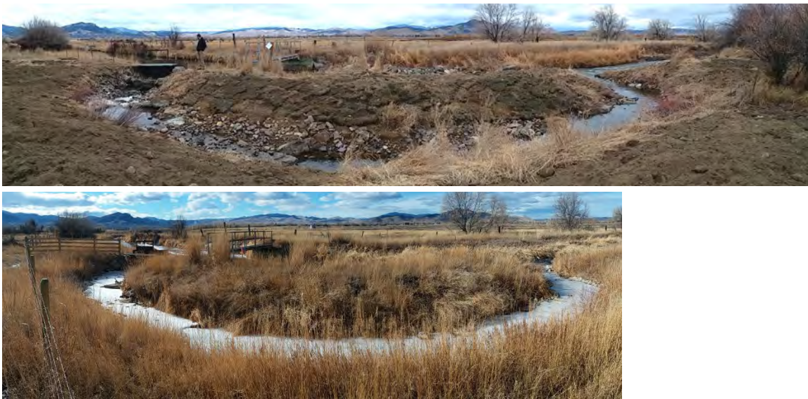
FIGURE 33. THE PRICKLY PEAR TRYAN FISH PASSAGE PROJECT AT PROJECT COMPLETION (TOP) AND IN 2021 (BOTTOM).
