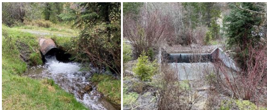
FIGURE 9. LITTLE PARK CREEK BARRIER BEFORE (L) AND AFTER (R) CONSTRUCTION. PHOTOS COURTESY OF THE CLARK FORK COALITION.
