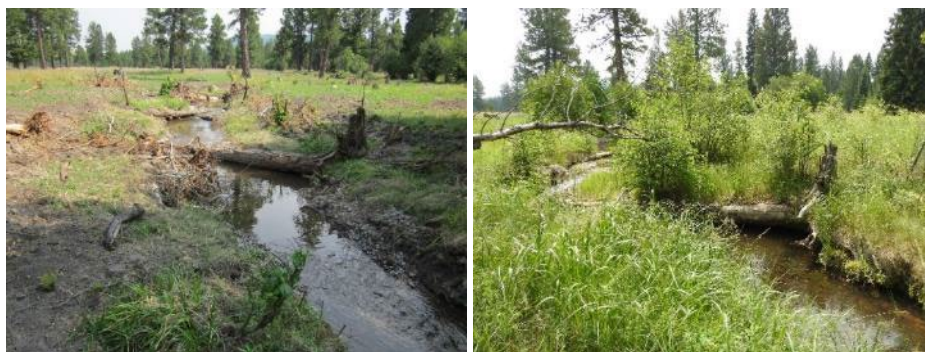
FIGURE 36. PEARSON CREEK AFTER CONSTRUCTION (2013) AND IN 2021. THE PHOTO VANTAGE POINT IS SIMILAR BETWEEN PHOTOS.
