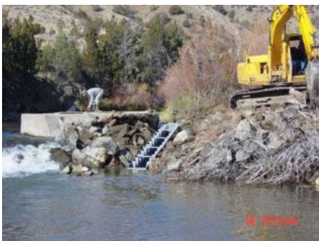
FIGURE 27. THE DENIL FISH LADDER, UPON INSTALATION. CURRENTLY THE LADDER IS IN DISREPAIR AND PARTIALLY FUNCTIONAL.
