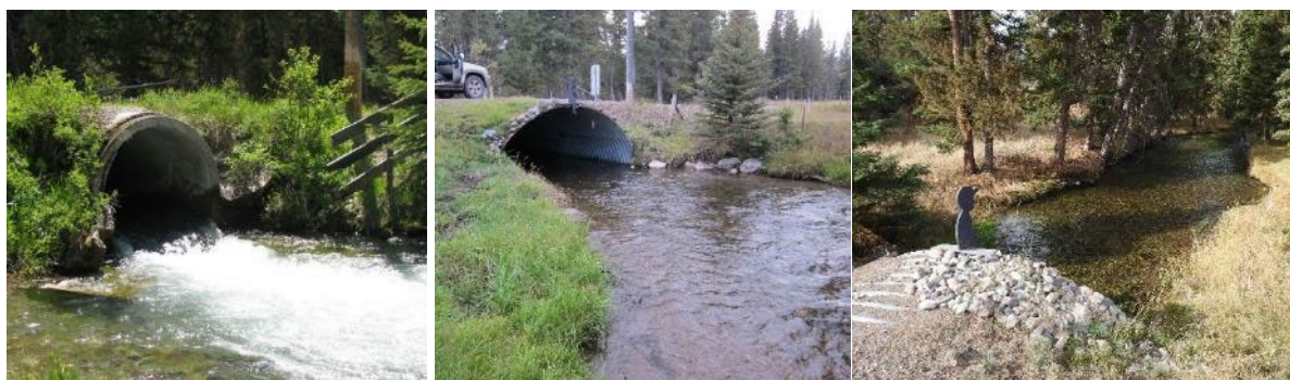
FIGURE 32. LINCOLN SPRING CREEK BEFORE (L) AND AFTER (MIDDLE) CONSTRUCTION, AND IN 2021 (R).
