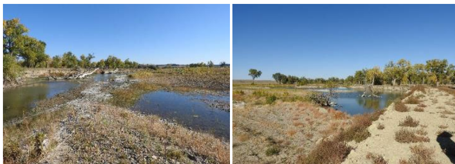
FIGURE 22. MUSSELSHELL RIVER MCCLEARY CHANNEL RESTORATION AFTER CONSTRUCTION, WHERE THE AVULSION OCCURED (L) AND CHANNEL PLUG (R).
