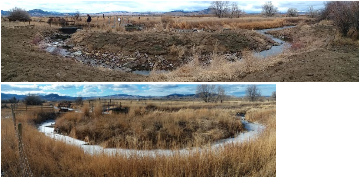
FIGURE 39. THE PRICKLY PEAR TRYAN FISH PASSAGE PROJECT AT PROJECT COMPLETION (TOP) AND IN 2021 (BOTTOM).
