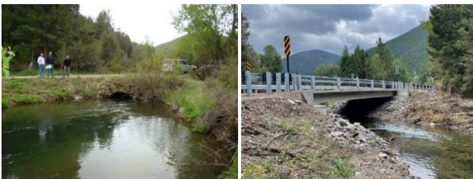
FIGURE 7. POORMAN CREEK CULVERT REPLACEMENT BEFORE (L) AND AFTER (R) CONSTRUCTION. PHOTOS COURTESY OF THE BIG BLACKFOOT CHAPTER OF TROUT UNLIMITED.
