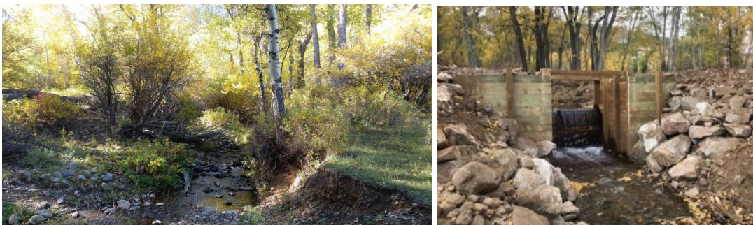
FIGURE 14. COTTONWOOD FISH BARRIER SITE BEFORE CONSTRUCTION (L) AND AFTER COMPLETION (R). PHOTOS COURTESY OF TROUT UNLIMITED AND FWP.
