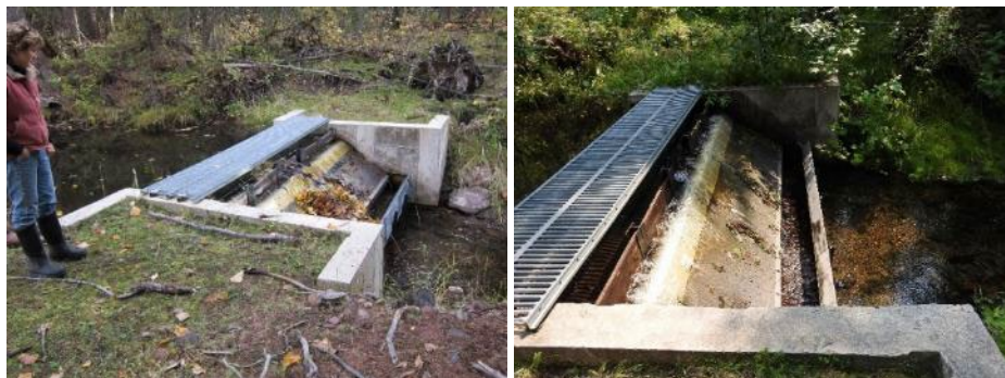
FIGURE 30. DICK CREEK FISH SCREEN IN 2011 (L) AND IN 2021 (R).
