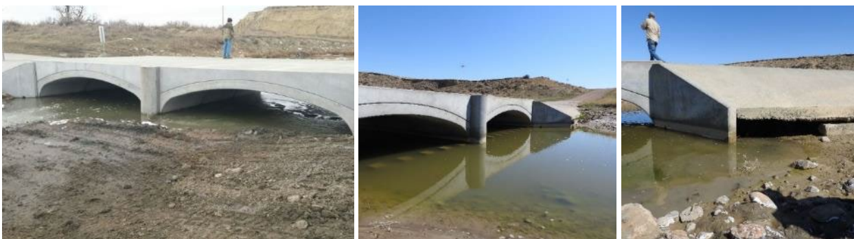
FIGURE 44. THE REDWATER RIVER NICKWALL CROSSING AFTER CONSTRUCTION (2016, L) AND IN 2021 (MIDDLE, R). NOTE THE EROSION OF THE WINGWALL TO BE REPAIRED IN 2021 (R).
