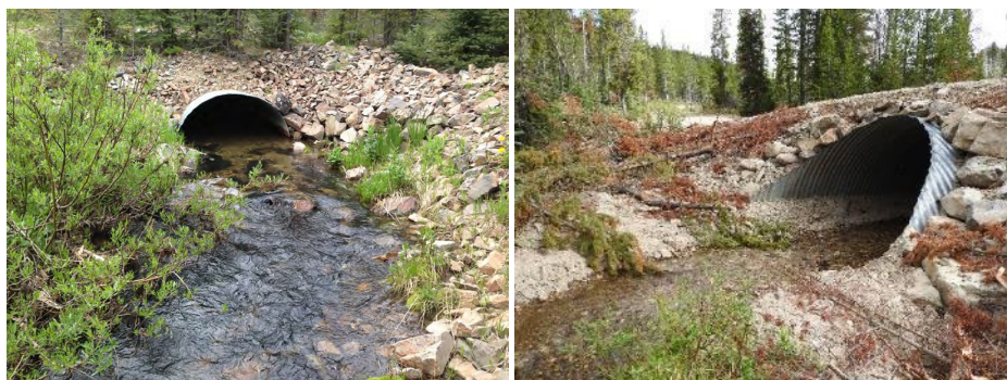
FIGURE 21. MONARCH CREEK CULVERT REPLACEMENT BEFORE (L) AND AFTER (R). PHOTOS COURTESY OF THE US FOREST SERVICE AND FWP.
