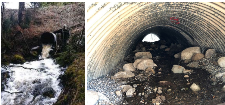
FIGURE 16. EAGLE CREEK CULVERT REPLACEMENT BEFORE (L) AND AFTER (R) CONSTRUCTION. PHOTOS COURTESY OF THE US FOREST SERVICE AND FWP.
