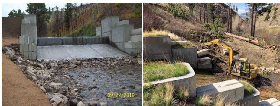
FIGURE 28. THE COTTONWOOD CREEK BARRIER AFTER CONSTRUCTION (2010, L) AND AS IT WAS REPAIRED IN 2021 (R).
