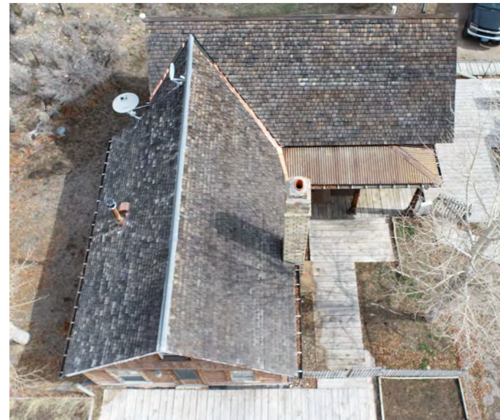
2 Manager's House - Roof Photo from the South Aerial Photograph - Not to Scale
