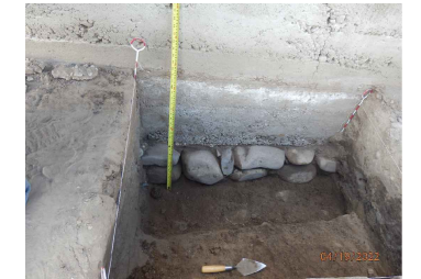
Photo of Representative Test Pit at East Wall Showing stone foundation and concrete plinth above
