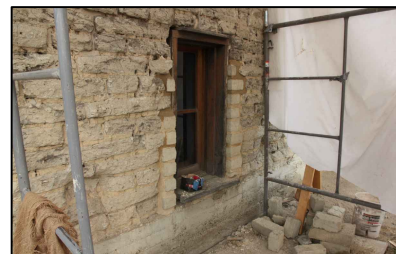
Photo of Representative Wall Area Exterior of Window into Room #100, at East Wall
