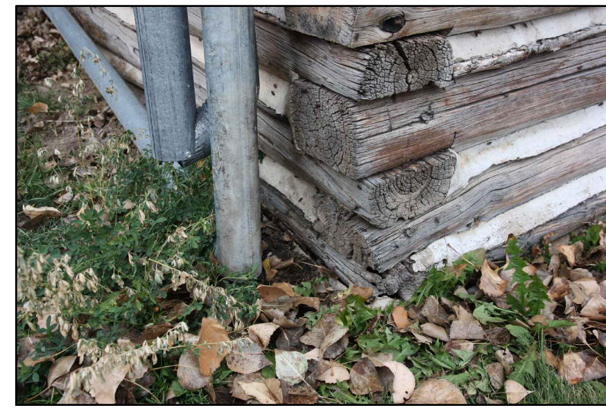
4 A3 CHIEF'S HOUSE DOWNSPOUT AT SOUTHWEST CORNER
