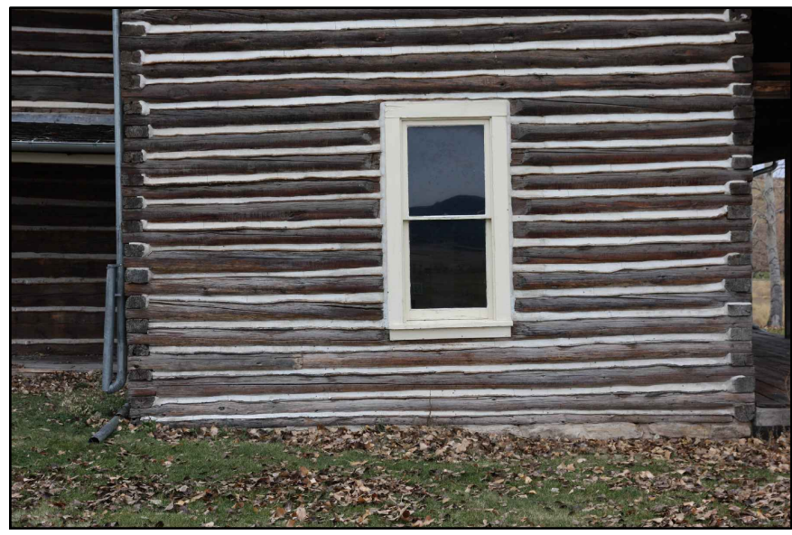
1 A3 CHIEF'S HOUSE SOUTHWEST CORNER WITH SETTLING
