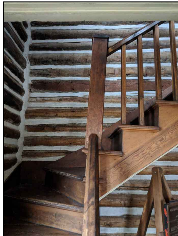
5 A3 CHIEF'S HOUSE SETTLING AT INTERIOR SOUTHWEST CORNER
