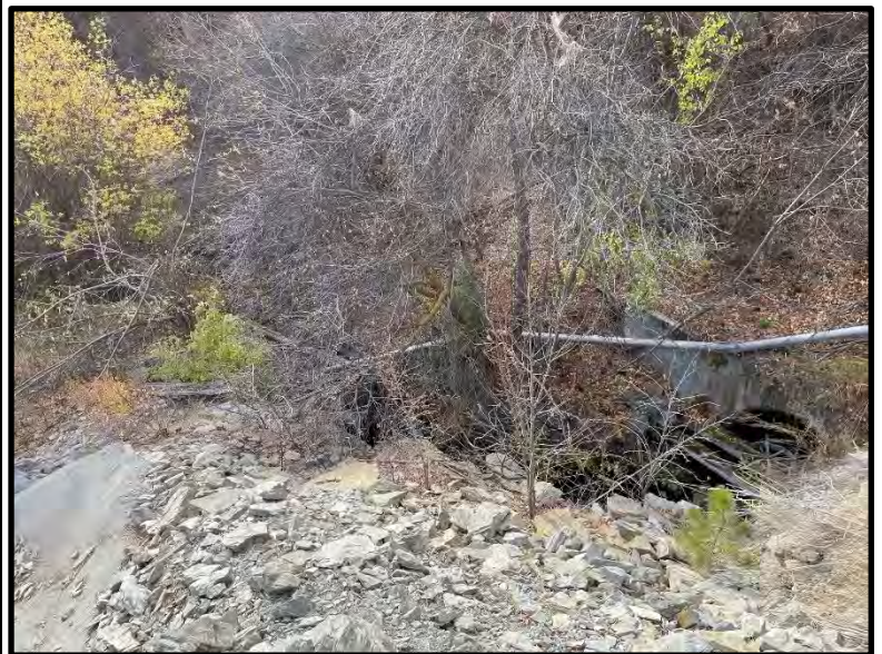
Drainage pipe discharge into outlet channel
