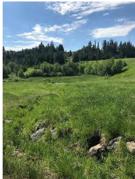
Figure 3. Existing bypass channel looking downstream to the dam outlet pipe in 2022. Note how the channel is filled in with vegetation.
