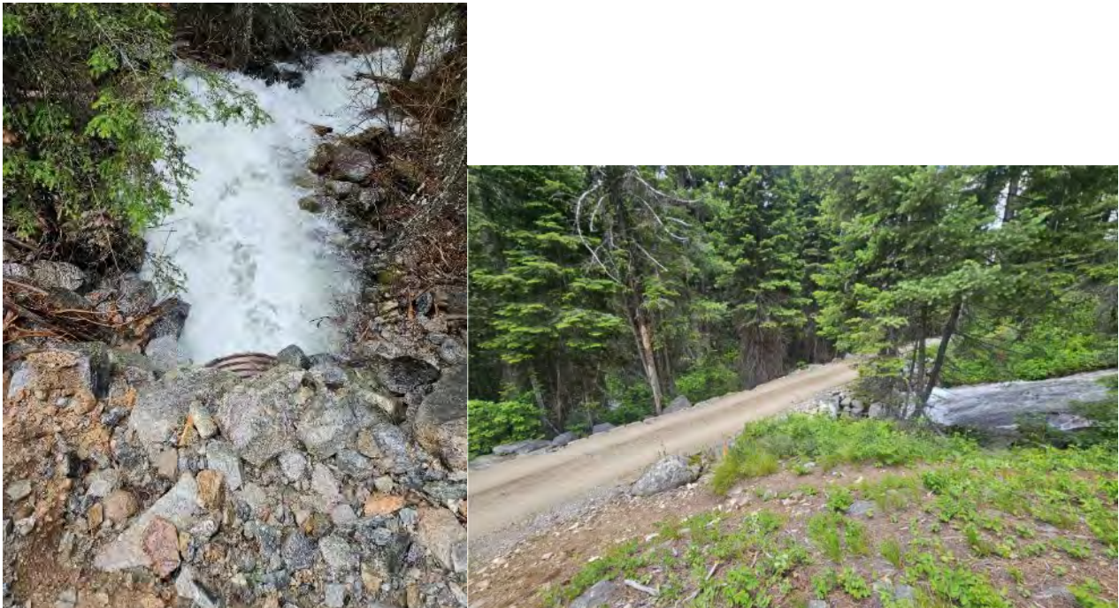
Left: The existing culvert, where a replacement bridge is proposed. Right: View from above of the Forest Road 429- Tenmile Creek crossing.
