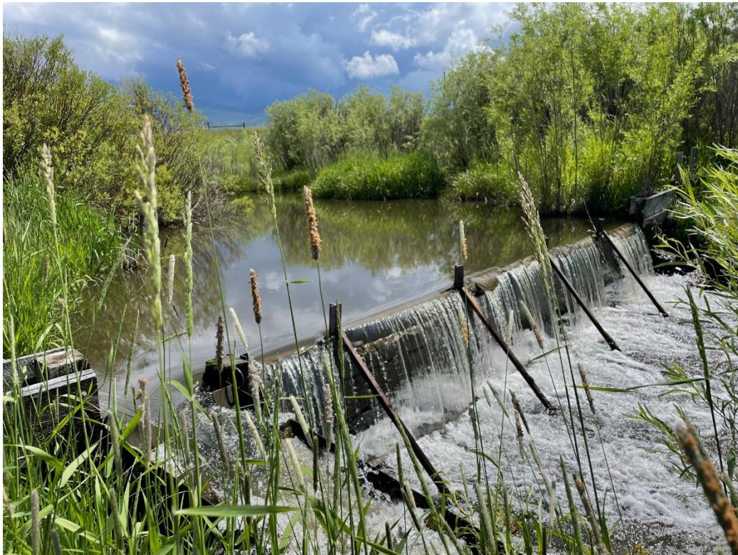
Photos 1 & 2: Existing Issues on Nevada Creek Phase 8
