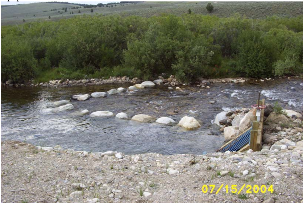
Photo 4G. The proposed diversion structure to replace and improve the current push up diversion structures found on the enrolled land of Landowner “A.” This “rock-vane” diversion is self-sustaining (no streambed disturbance apart from installation) and allows fish passage.
