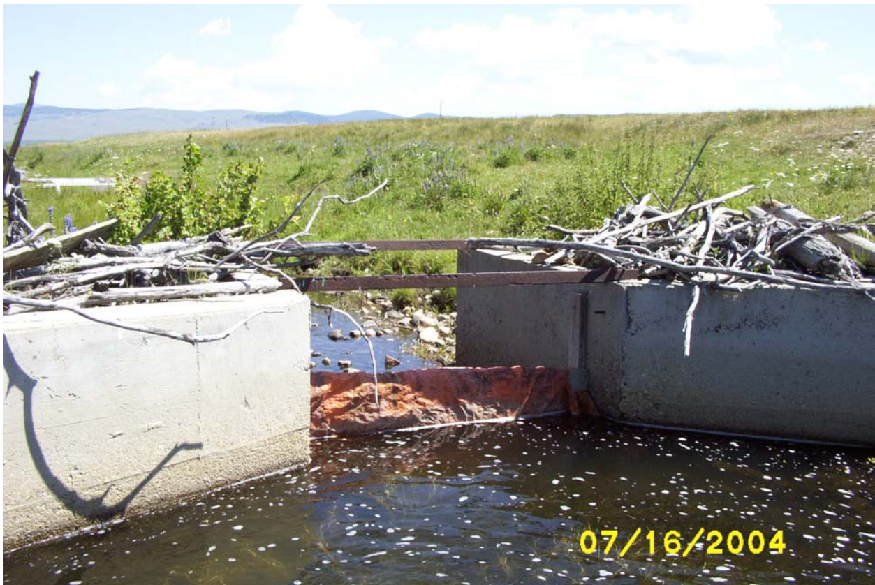
Photo 2G. The current condition of a headgate on the enrolled land of Landowner “A.”
