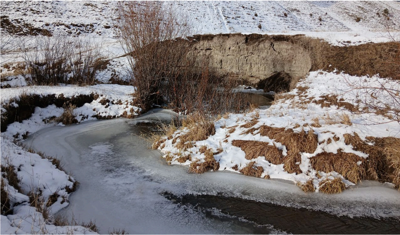
Photo 5, Unit 1: 10-foot tall, eroded bank.
