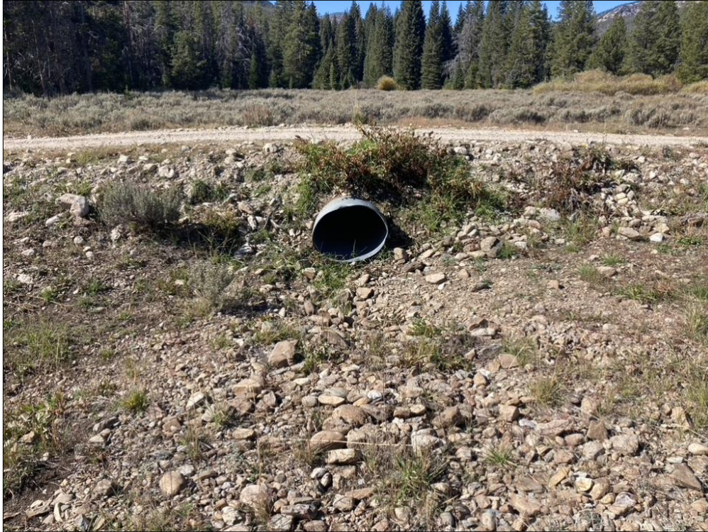
Figure 3. Looking upstream, 45.16963, -113.5206, One of two (southern) undersized culverts is to be removed and the road obliterated.
