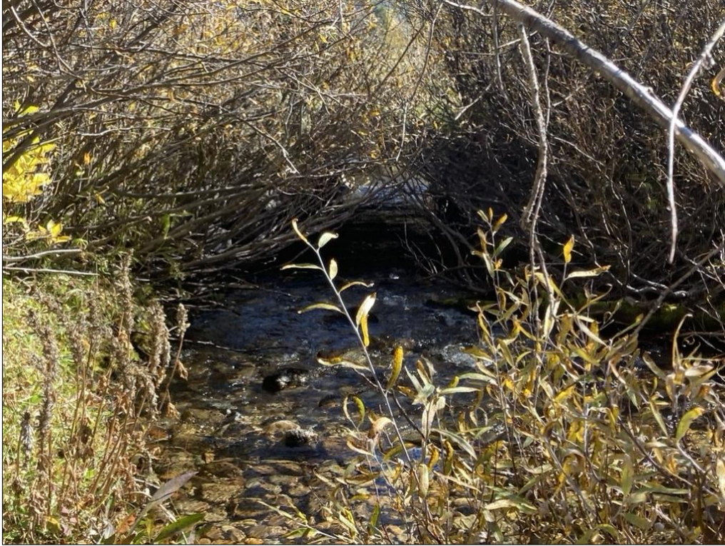
Looking downstream at Darkhorse Creek, 45.17006, -113.52083. One of two (northern) undersized culverts is to be removed and the road obliterated.
