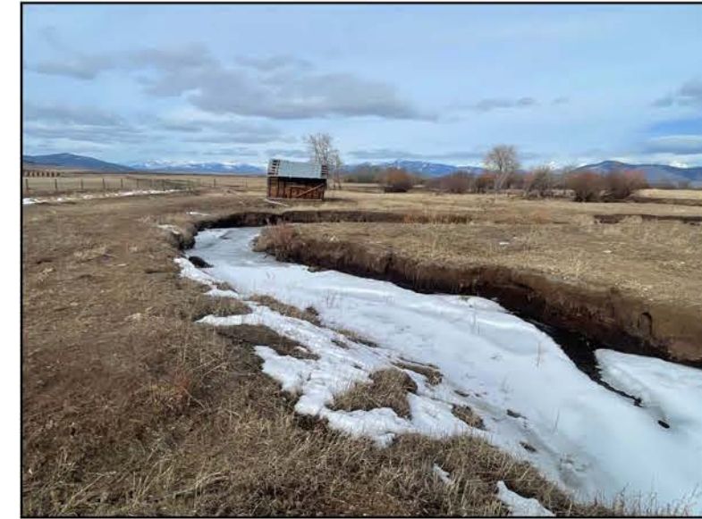
HIGH BANK HEIGHT RATIOS AND CHANNEL ENTRENCHMENT DRIVES EROSION IN REACH 2 . VEGETATION COMMUNITIES HAVE CONVERTED FROM A LIKELY WOODY RIPARIAN COMMUNITY TO A GRASS/FORB AGRICULTURAL ASSEMBLAGE.
