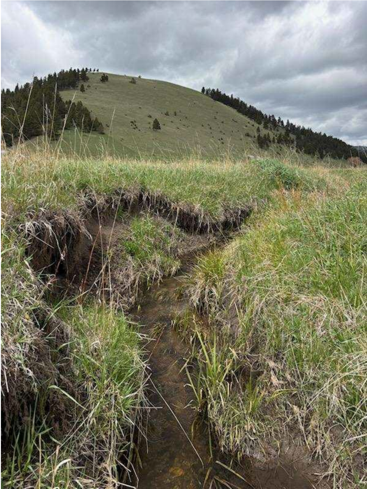
Figure 2. Photograph of incised channel on Marsh Creek within the proposed restoration area.
