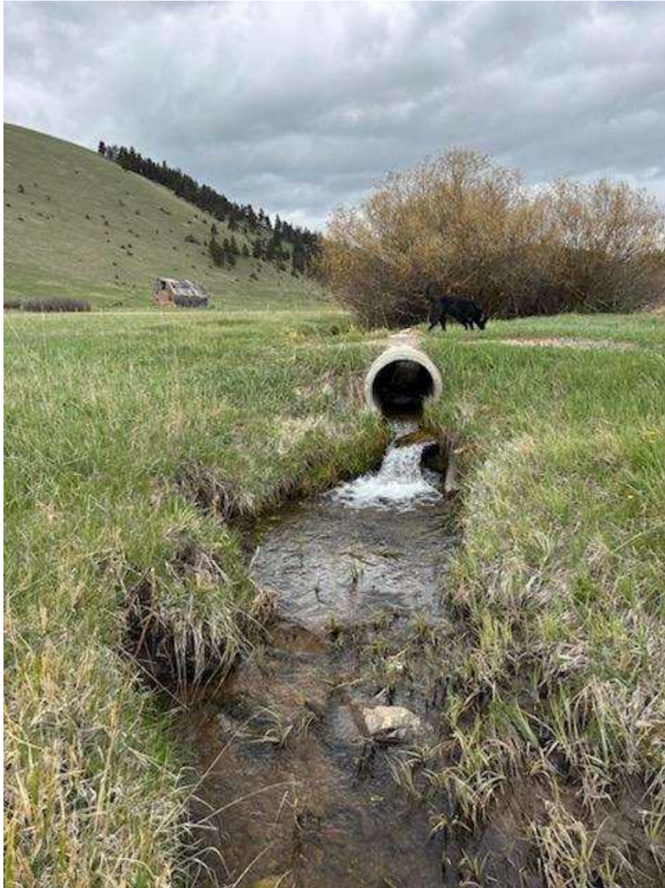
Figure 3. Photograph of perched culvert on Marsh Creek within the proposed project area.
