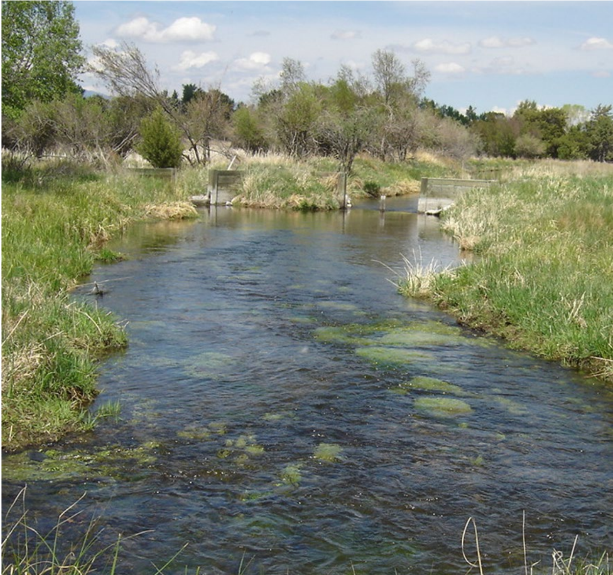
Figure 2. A view looking downstream at the irrigation diversion structure on Parsons Slough below Loomont Lane. The gate on the left controls flow to the spawning channel that joins the Jefferson River. The larger gate on the right controls flow to the irrigation ditch. The proposed project will eliminate the need to divert any water at this location.
