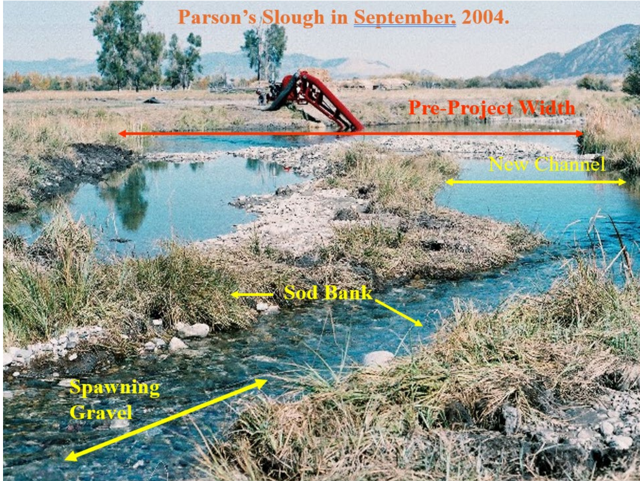
Figure 15. Habitat restoration work on Parsons Slough to improve water conveyance, fish passage, and trout spawning and rearing.
