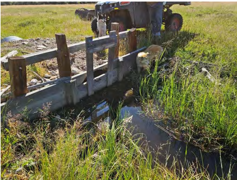
Old slide gate that does not function.
