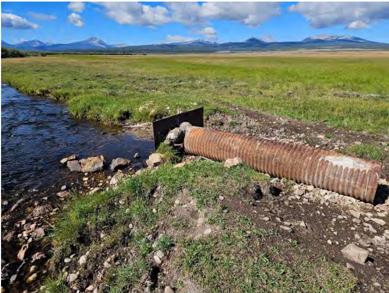
Old pipe for the ditch that is no longer aligned with the ditch.
