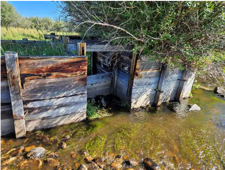
Old pin and plank on the ditch entrance.
