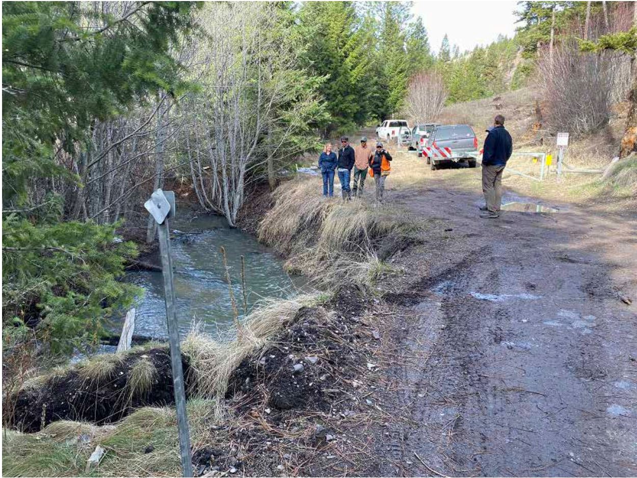
Figure 1. O'Brien Creek is eroding the stream-side roadbed at several locations. This picture shows an actively eroding section of roadbed the at the beginning of the restoration reach. The road will be re-located away from the stream, and vegetated wood matrix and large wood structures will be installed creating an inset floodplain.
