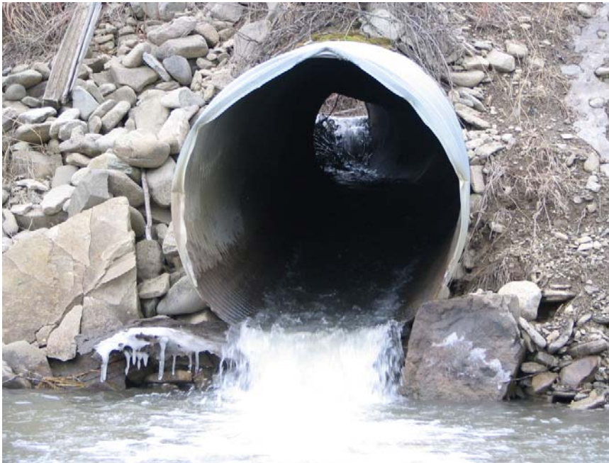
Figure 4-1: Culvert presenting a probable fish barrier on the lower end of the Brumfield property.
