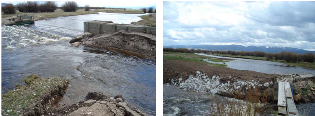
Figure 3. The breach in the Spokane Irrigation Ditch caused by ice jams and the repair made to insure water could be properly managed at this point of diversion (project photos).
