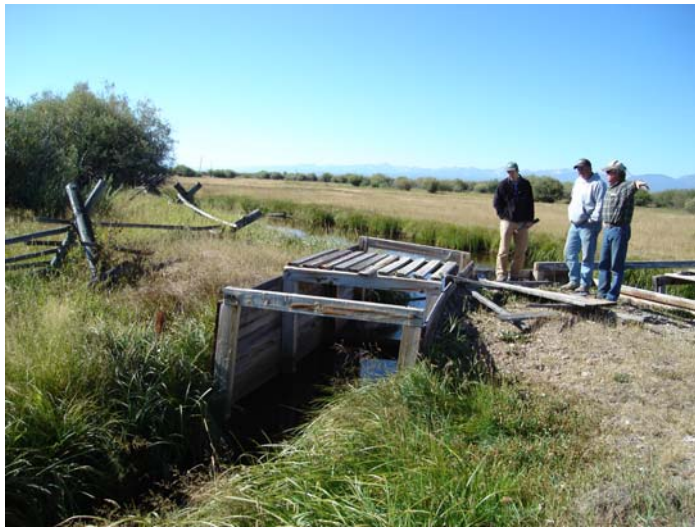
Figure 5. One of the headgates to be replaced as part of the Huntley Irrigation Improvement Project (pre-project photo).
