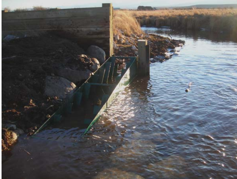
Figure 24. A denil-style fish ladder installed in an irrigation diversion in Rock Creek to provide passage to migratory fish (project photo)
