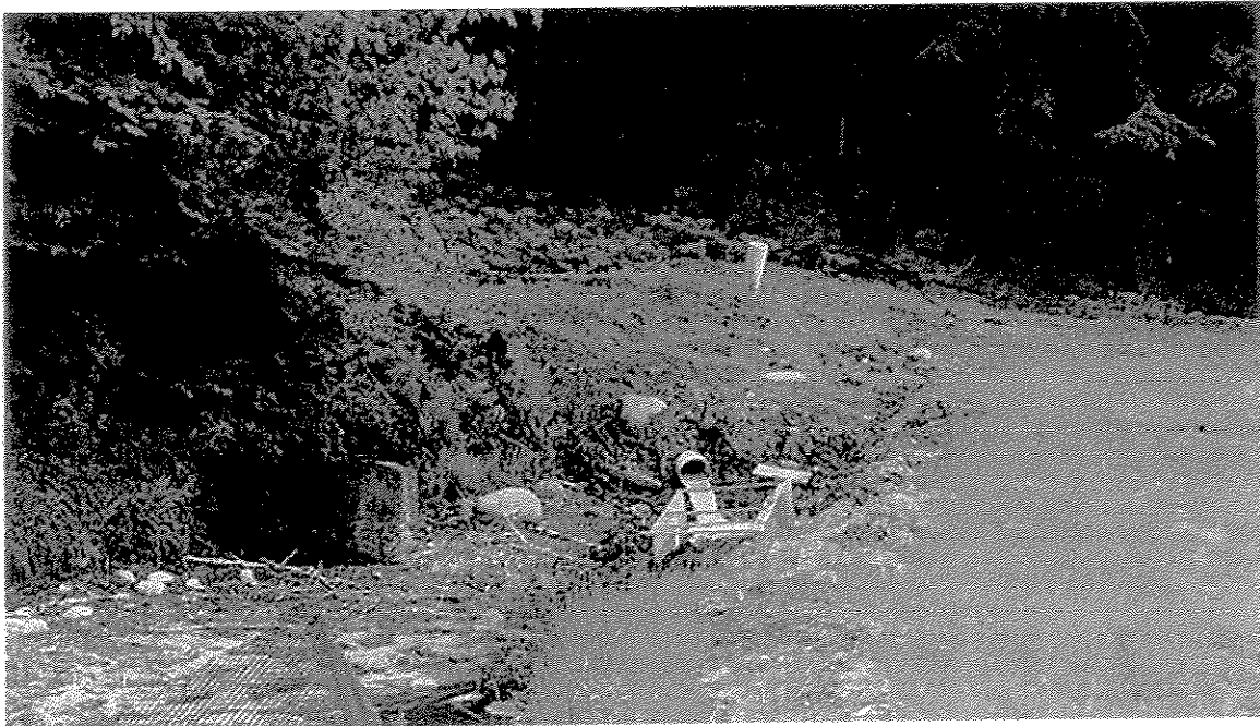
Figure 11. Spring #2 after preliminary revegetation to stabilize the site. Additional vegetation will be added after the stream channel is restored.
