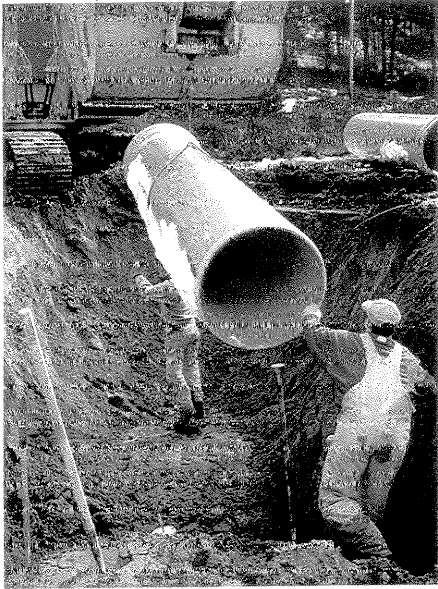
Figure 3. Replacement of the culvert leading from the former head pond to the lower stream reaches.
