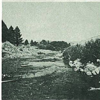
Flint Creek in 1957 near junction of 10A and No. 38. New highway construction. Channel cleared and straightened by bulldozer.
