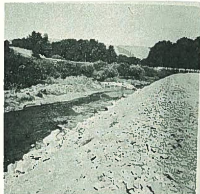
Flint Creek near junction of U. S. 10A and No. 38. New highway construction
