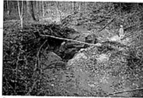
Severe stream bank erosion
