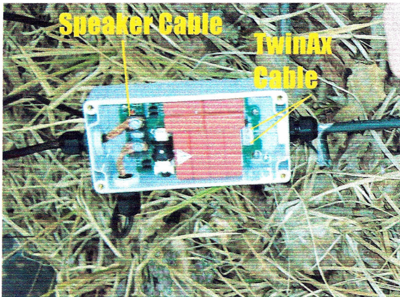
Figure 3. Cable connections inside the remote tuner box showing proper wiring. FWP photo.
