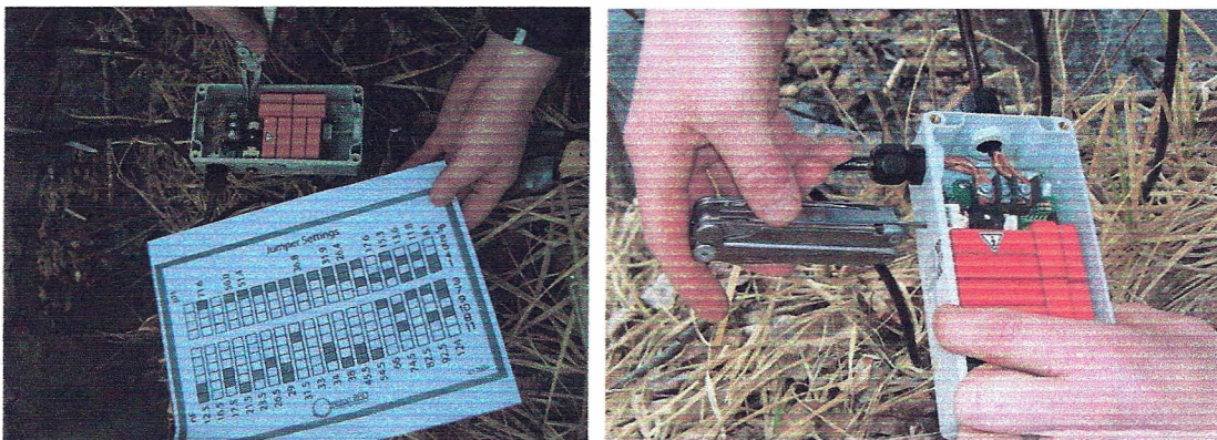
Figure 6a. Adjusting settings in the remote tuner box by moving jumpers; and 6b. Fine tuning the remote tuner box using a small screwdriver.
