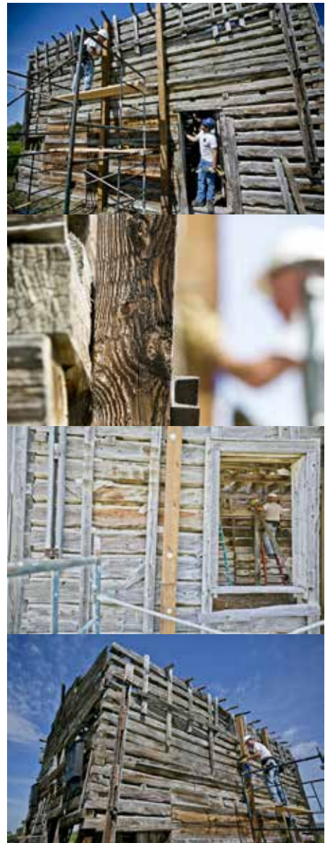
Stabilizing of Gallatin City Hotel at Missouri Headwaters State Park by park staff and consultant Kirby Matthew. Photo by Adrian Sanchez-Gonzalez / Bozeman Daily Chronicle.
