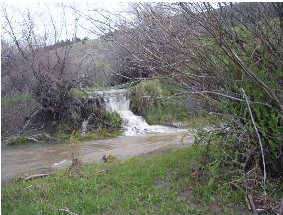
Figure 2-89. Head cut on South Fork Horse Creek caused by flood.
