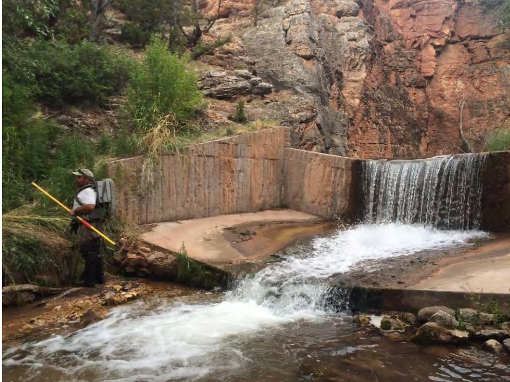
Figure 2-23. Downstream end of apron showing lack of a plunge pool.
