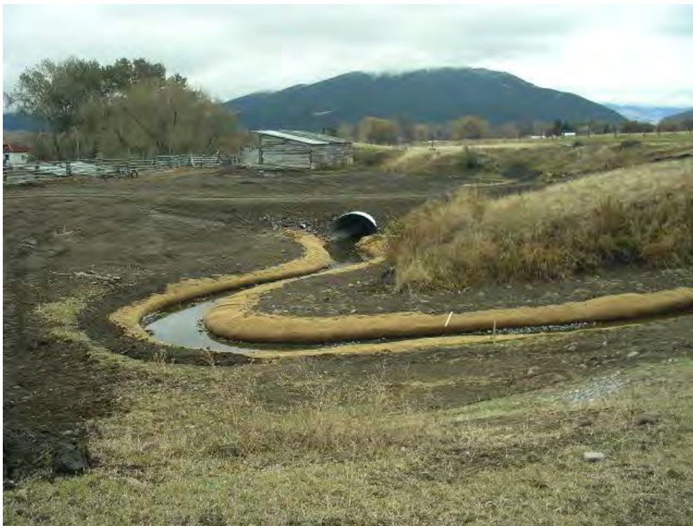
Figure 2-50. Example of newly constructed channel on Fleshman Creek and stream crossing with bottomless arch culvert and overflow pipes.
