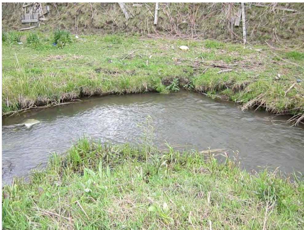
Figure 2-53. Outer meander bend showing stable bank constructed with coir fabric encapsulated soil lifts. (Note that photo was taken in early June, and ground cover was beginning to grow for the season.)
