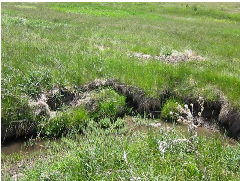
Photo 3: Sloughing of stream bank.
