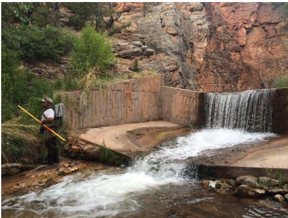
Photo 3. Slight amount of scour at downstream of apron, but not deep enough to allow to leap.
