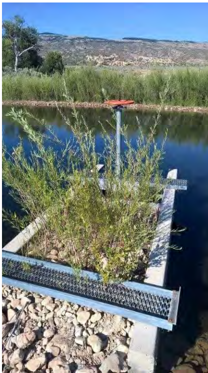
Photo 3. Willows growing on one of the irrigation stand pipes
