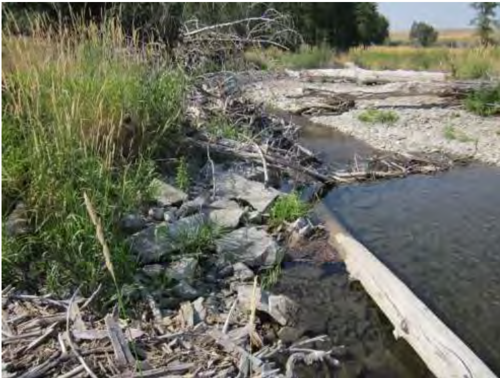
Figure 66. Bank armoring and large woody debris.
