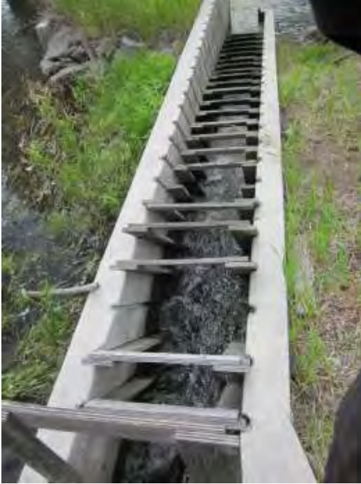
Figure 91. Denil fish ladder on South Fork Fridley Creek.
