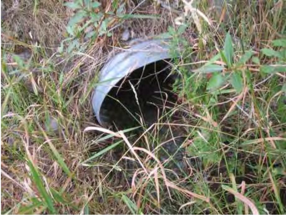
Figure 24. Inlet of pipe that passes the unnamed spring creek under the corrals adjacent to Elk Creek.
