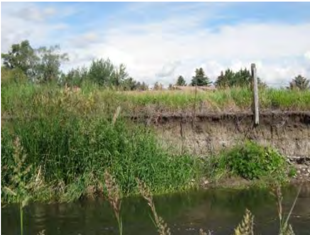
Figure 21. Vertical exposed stream bank and evidence of lateral movement, as indicated by the hanging fence post.
