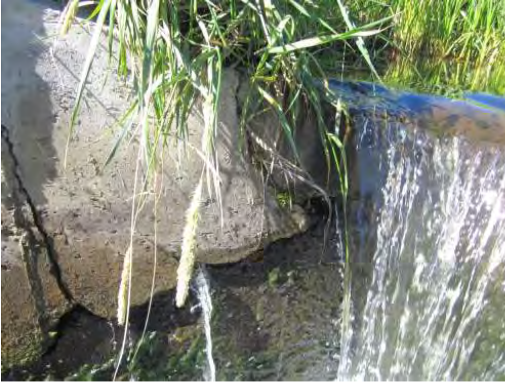
Figure 104. Crumbling concrete on right side of barrier.
