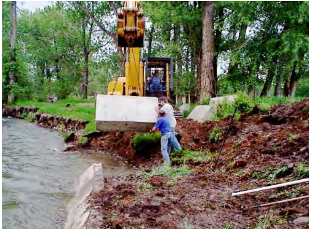
Figure 60. Project construction photo showing existing eroding bank from a PowerPoint presentation prepared in 2002.
