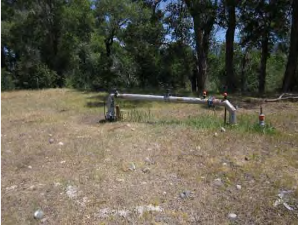
Figure 34. Pumping station supplying water to center pivots.
