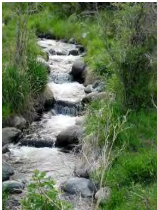
Figure 28. Step/pool sequence constructed upstream of the culvert diverting North Fork Fridley Creek under the Park Branch Canal, to match pre-project grade and provide fish passage from the Yellowstone River.
