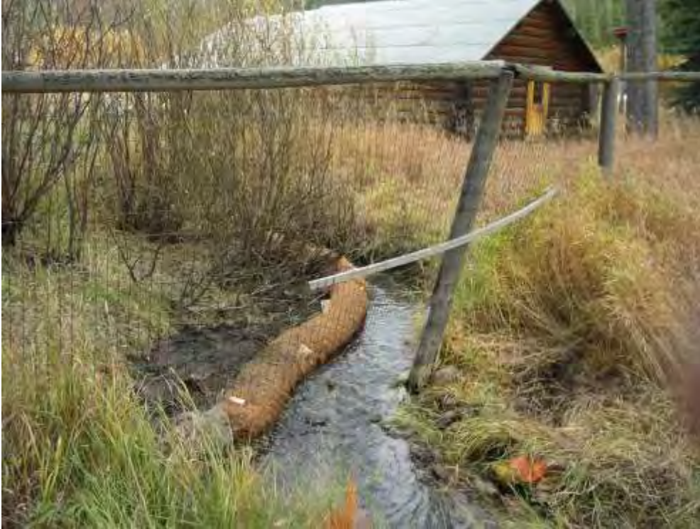
Figure 114. New bank built with straw wattle and back filled with sediment excavated from channel.
