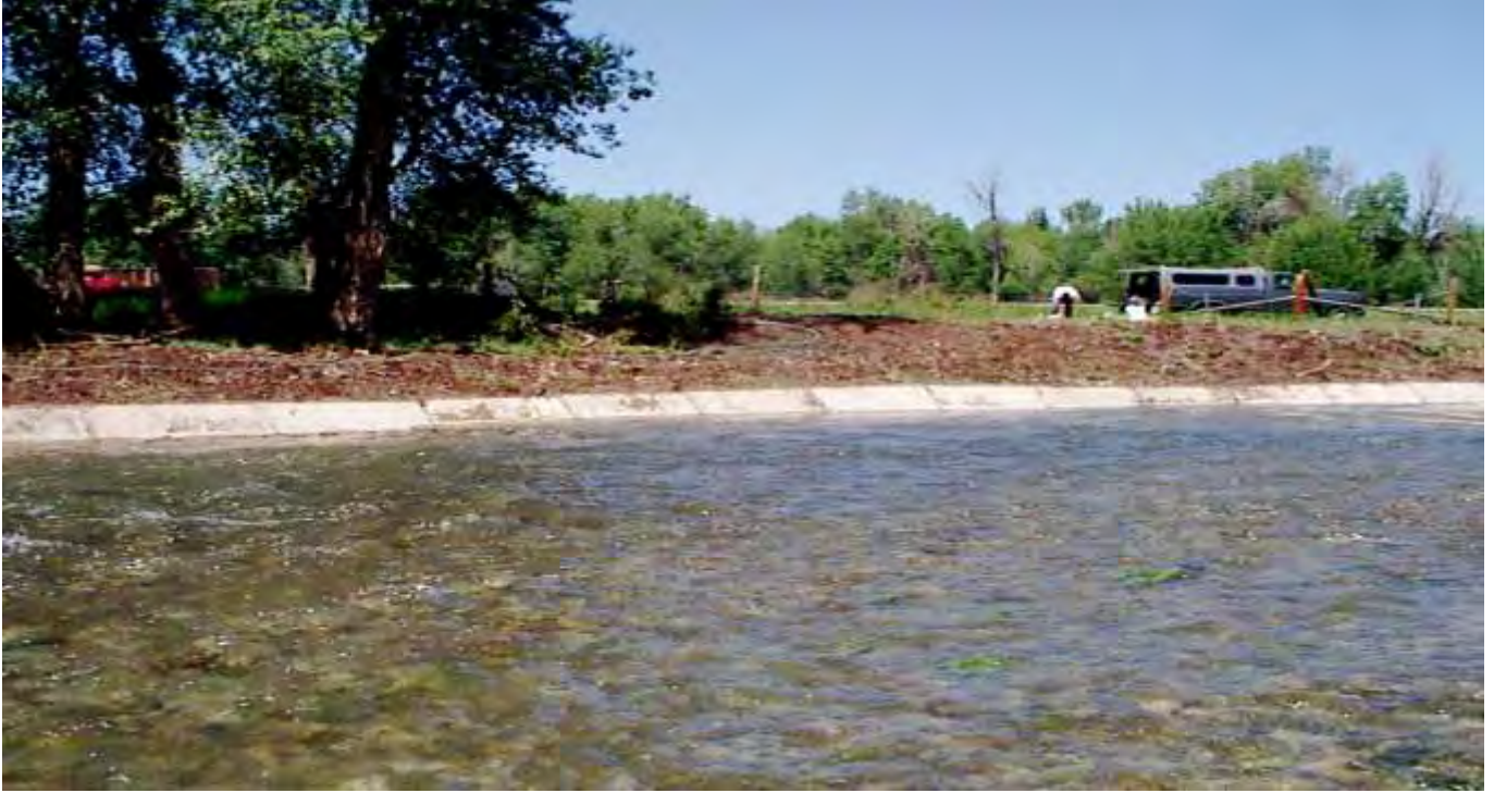
Figure 61. Concrete blocks installed along the bank line from a PowerPoint presentation prepared in 2002.
