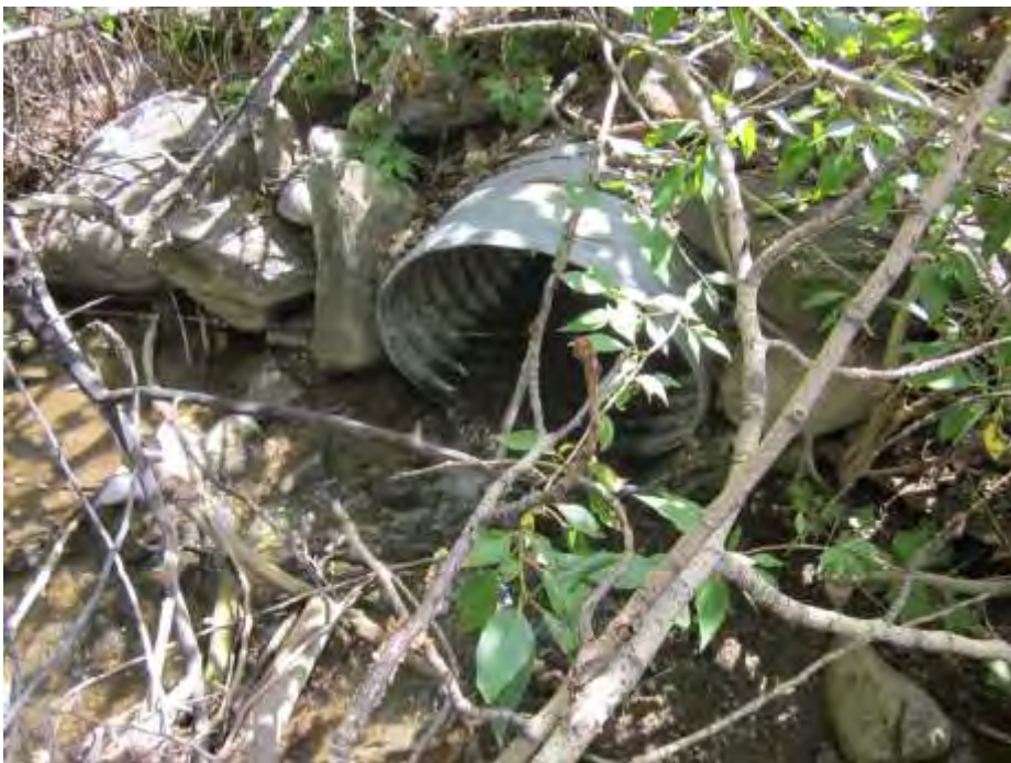
Figure 25. Outlet of pipe that passes the unnamed spring creek under the corrals adjacent to Elk Creek.
