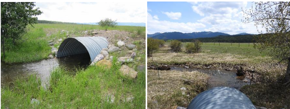
FIGURE 101. ROCK CREEK CULVERT IN 2013 (L) AND 2019 (R). THE CULVERT IS INTACT BUT THERE IS SOME DOWNSTREAM EROSION.
