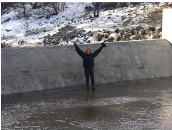
FIGURE 51. LOWER DEER CREEK AFTER CONSTRUCTION AS WATER WAS FILLING BEHIND THE STRUCTURE.
