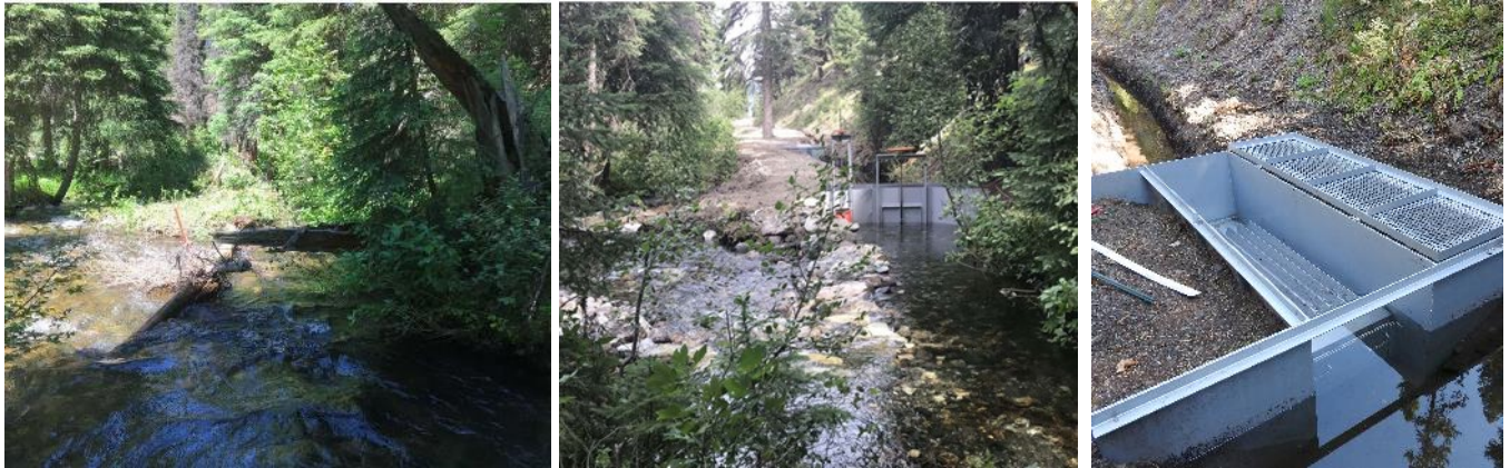
FIGURE 17. WILSON DITCH BEFORE (L) AND AFTER (CENTER) AFTER DIVERSION UPGRADE. PHOTOS COURTESY OF TROUT UNLIMITED. A CORRUGATED WATER FISH SCREEN WAS INSTALLED IN THE DITCH (R).
