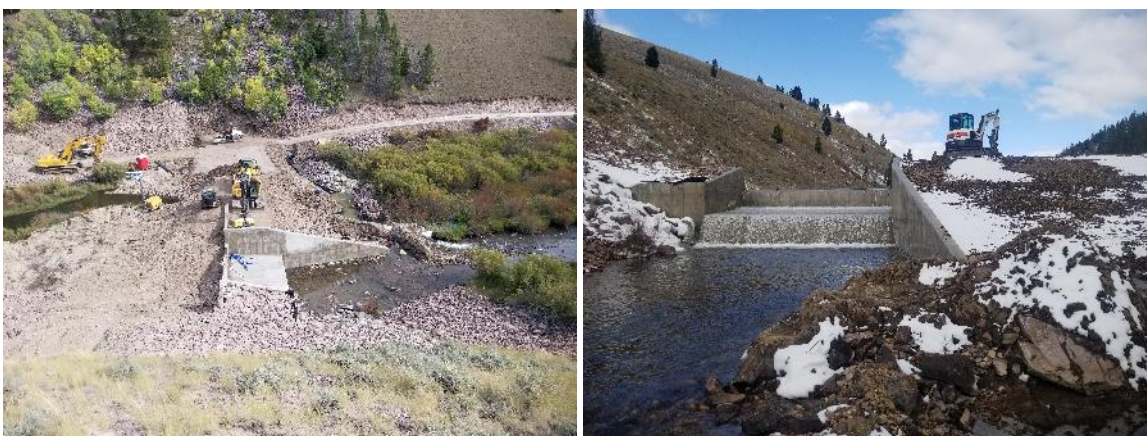
FIGURE 29. FRENCH CREEK BARRIER IN CONSTRUCTION (L) AND AFTER COMPLETION (R). THE NEXT PHASE OF THIS PROJECT WILL BE TO REMOVE NON-NATIVE FISH AND REINTRODUCE ARCTIC GRAYLING AND WESTSLOPE CUTTHROAT TROUT.
