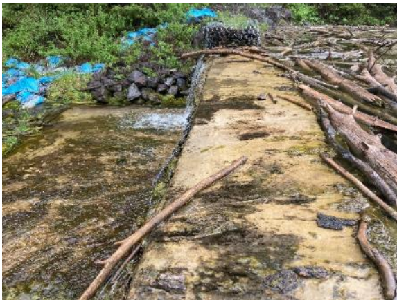
FIGURE 49. TOP OF LAKE CREEK FISH BARRIER SHOW WEAR AND ACCUMULATIONS OF WOODY DEBRIS.
