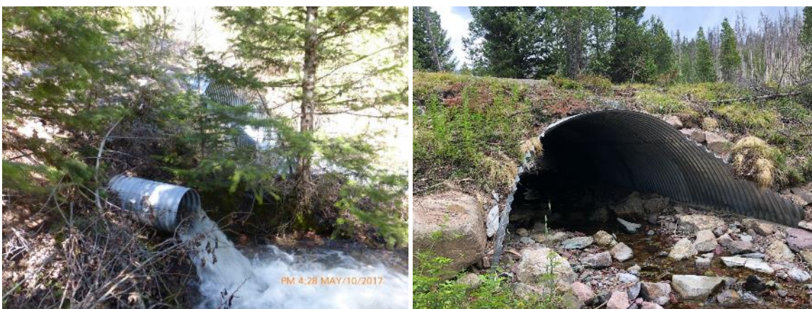
FIGURE 40. THIS PROJECT, ON NORTH FORK KEEP COOL CREEK, REPLACED AN UNDERSIZED CULVERT THAT WAS A BARRIER AT MOST FLOWS (L) WITH A LARGER CULVERT THAT IMPROVES FISH PASSAGE AND CONNECTIVITY (R). BEFORE PHOTO COURTESY OF BIG BLACKFOOT CHAPTER OF TROUT UNLIMITED.
