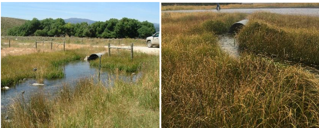
FIGURE 90. MADISON SPRING CREEK IN 2009 (L) AND 2020 (R). THE STREAM HAS ADJUSTED BUT THE RIPARIAN AREA IS IN GOOD CONDITION.
