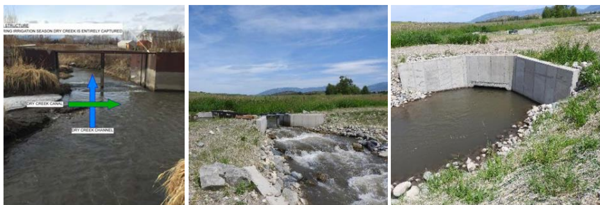
FIGURE 28. DRY CREEK FISH PASSAGE BEFORE RESTORATION (L), WHERE THE CREEK WAS INTERCEPTED BY THE DITCH. THE PROJECT INSTALLED NEW IRRIGATION INFRASTRUCTURE (MIDDLE) AND BUILT A CULVERT TO ROUTE THE STREAM UNDERNEATH THE DITCH (R). BEFORE PHOTO COURTESY OF TROUT UNLIMITED.
