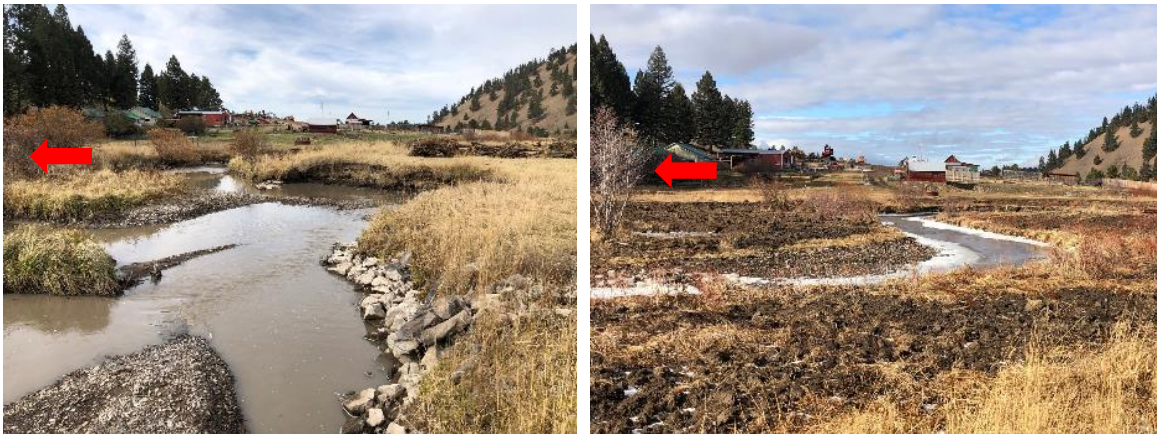
FIGURE 7. NEVADA CREEK BEFORE (L) AND AFTER (R) CONSTRUCTION. PHOTOS COURTESY OF BIG BLACKFOOT CHAPTER OF TROUT UNLIMITED. THE RED ARROW IS FOR REFERENCE POINT IN BOTH PHOTOS.
