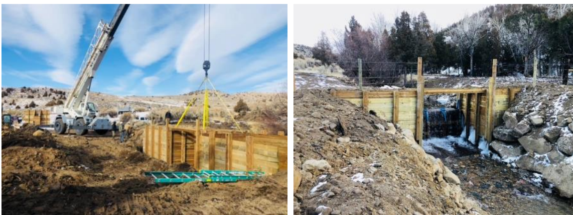
FIGURE 42. THE RAMSHORN CREEK FISH BARRIER DURING CONSTRUCTION (L) AND AFTER COMPLETION (R).
