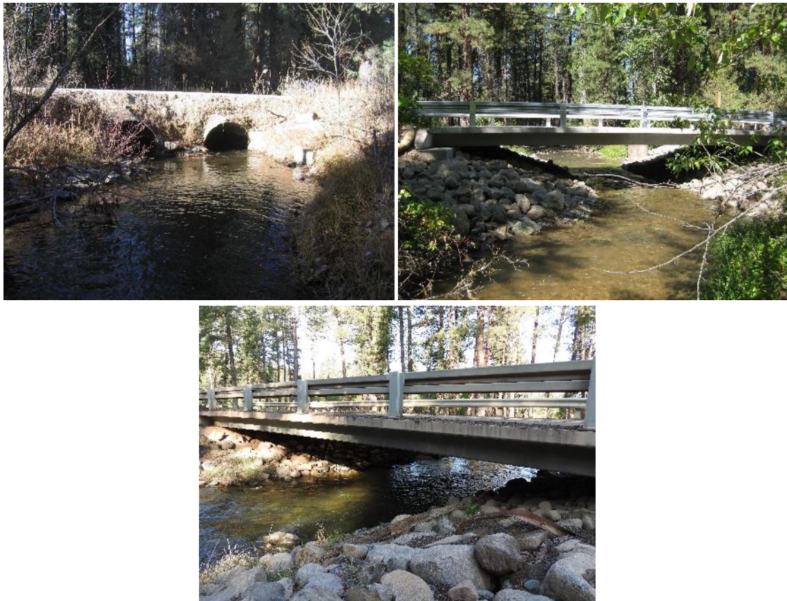
FIGURE 94. POORMAN CREEK BEFORE (TOP LEFT) AND AFTER CONSTRUCTION (TOP RIGHT; 2009). THE BRIDGE WAS IN GOOD CONDITION IN 2020 (BOTTOM).
