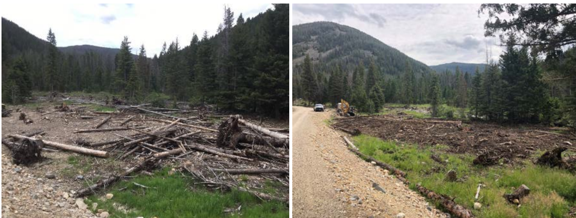
FIGURE 33. ONTARIO CREEK WAS AFFECTED BY MANY ROADS WITHIN THE FLOODPLAIN (L). THIS PROJECT DECOMMISSIONED THE UNAUTHORIZED ROADS AND MOVED THE MAIN ROAD OUT OF THE FLOODPLAINS. PHOTOS COURTESY OF THE U.S. FOREST SERVICE.
