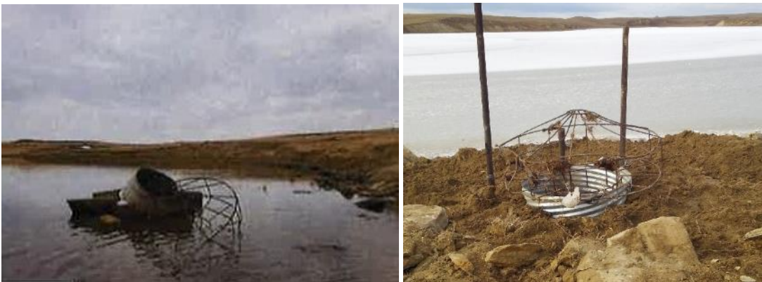
FIGURE 12. HAUGHIAN RESERVOIR SPILLWAY PIPE BEFORE (L) AND AFTER (R) CONSTRUCTION. BEFORE PHOTO COURTESY OF PAT HAUGHIAN.
