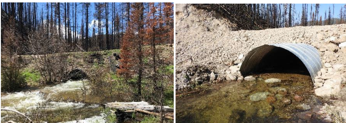
FIGURE 31. AN UNDERSIZED CULVERT IMPAIRED FISH PASSAGE ON GREEN CANYON CREEK (L) AND WAS REPLACED WITH A LARGER CULVERT (R). BEFORE PHOTO BY TROUT UNLIMITED.
