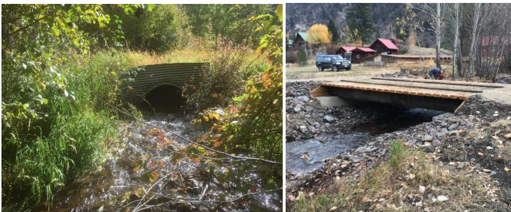
FIGURE 23. BREWSTER CREEK BEFORE (L) AND AFTER (R) RESTORATION. AN UNDERSIZED CULVERT WAS REPLACED WITH A FARM BRIDGE. PHOTOS COURTESY OF TROUT UNLIMITED.
