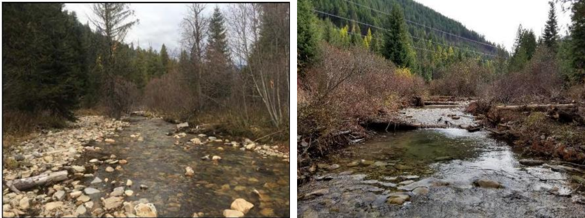
FIGURE 6. CROW CREEK BEFORE (L) AND AFTER (R) CONSTRUCTION. PHOTOS COURTESY OF LOWER CLARK FORK WATERSHED GROUP AND RIVER DESIGN GROUP. NOTE HABITAT STRUCTURE ADDED TO THE RIGHT SIDE OF THE AFTER PHOTO.
