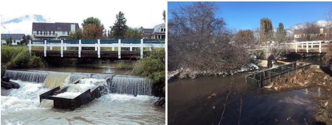
FIGURE 35. MILL CREEK FISH LADDER BEFORE (L) AND AFTER IT WAS REPLACED FOR FUNCTIONALITY (R). AFTER PHOTO COURTESY OF TROUT UNLIMITED.
