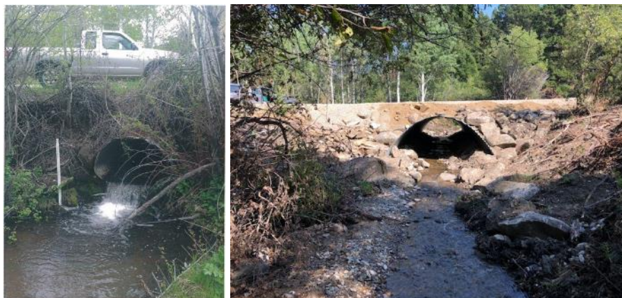
FIGURE 38. AN UNDERSIZED CULVERT ON NORTH FORK DRY COTTONWOOD CREEK (L) WAS REPLACED WITH A LARGER ARCH CULVERT FOR FISH PASSAGE (R). BEFORE PHOTO COURTESY OF CLARK FORK COALITION.
