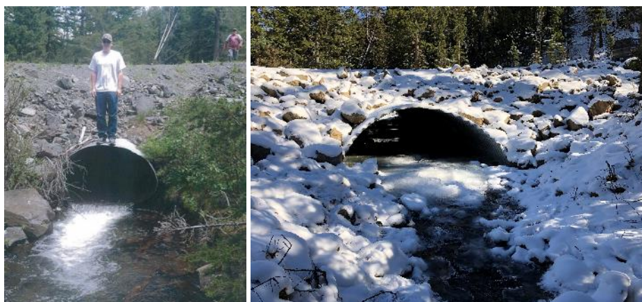
FIGURE 37. NORTH FORK COTTONWOOD CREEK HAD AN UNDERSIZED CULVERT (L) THAT WAS REPLACED WITH A LARGER CULVERT (R), WHICH ENHANCED FISH PASSAGE AND STREAM FUNCTION. BEFORE PHOTO COURTESY OF CLARK FORK COALITION.
