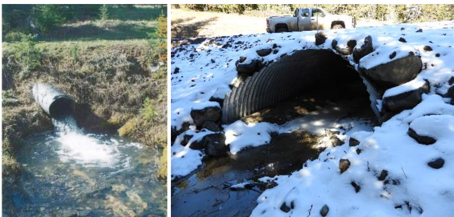
FIGURE 43. THIS PROJECT ON TURKEY CREEK REPLACED AN UNDERSIZED CULVERT (L) WITH A LARGER CULVERT THAT PROVIDES CONNECTIVITY AND FISH PASSAGE (R). BEFORE PHOTO COURTESY OF THE U.S. FOREST SERVICE.
