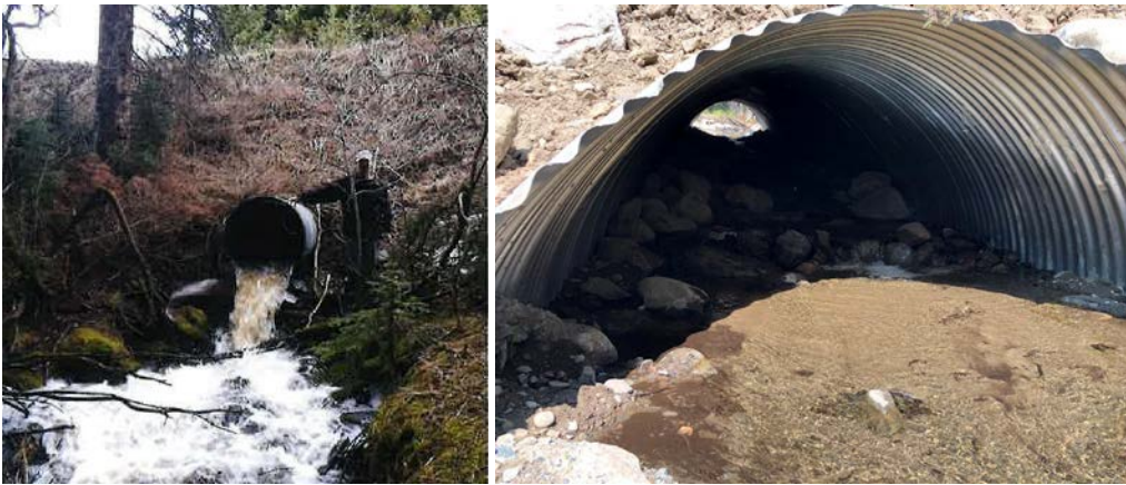
FIGURE 19. EAGLE CREEK UNDERSIZED CULVERT BEFORE CONSTRUCTION (L) AND LARGER ARCH CULVERT (R) AFTER CONSTRUCTION. BEFORE PHOTO COURTESY OF THE U.S. FOREST SERVICE.
