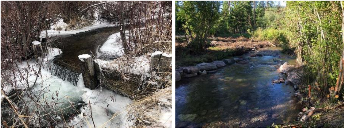
FIGURE 18. BOLES CREEK DIVERSION BEFORE CONSTRUCTION (L) AND AFTER CONSTRUCTION (R), USING A ROCK CROSS-VANE TO DIVERT WATER AND MAINTAIN FISH PASSAGE. BEFORE PHOTO COURTESY OF BIG BLACKFOOT CHAPTER OF TROUT UNLIMITED.
