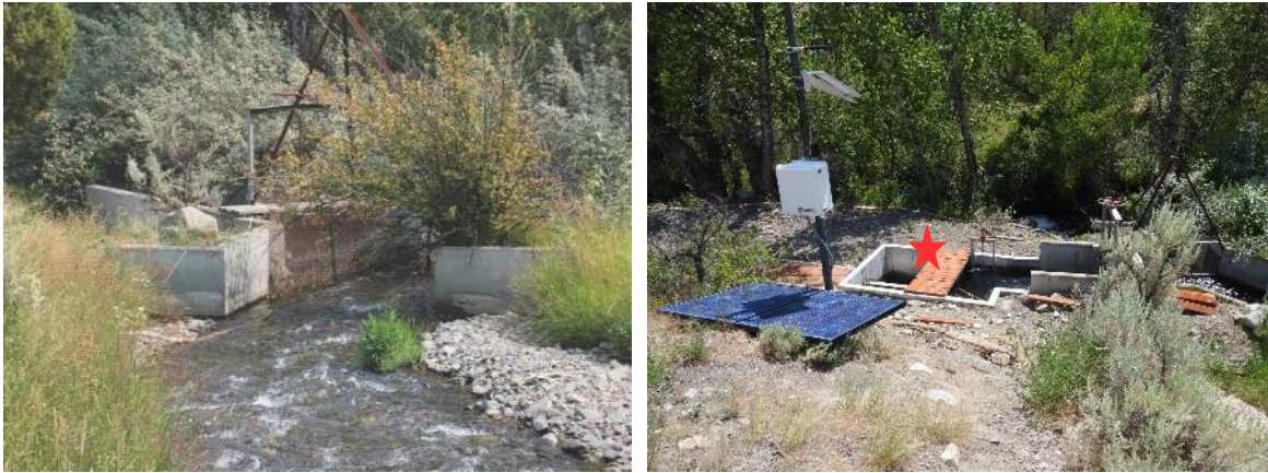
FIGURE 16. REESE CREEK DIVERSION BEFORE (L) AND AFTER (R) RESTORATION. THE PROJECT INCLUDED INSTALLATION OF A FISH SCREEN AND PIPELINE (DENOTED BY STAR). BEFORE PHOTO COURTESY OF TROUT UNLIMITED.
