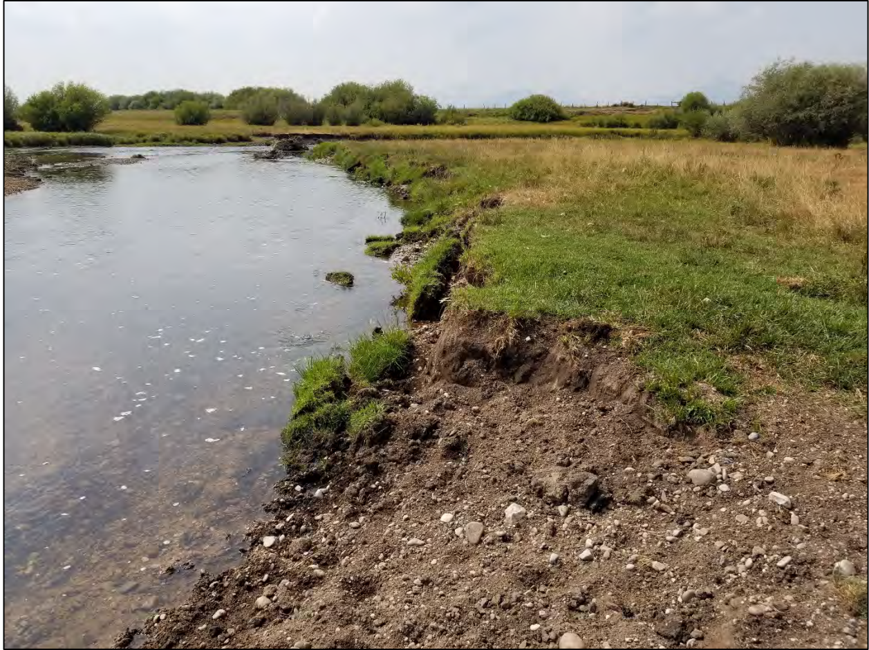
Streambank prior to temporary fix.
