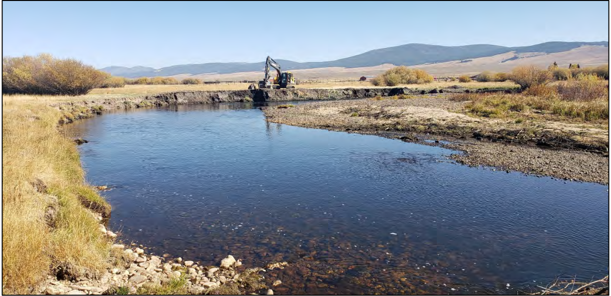
Streambank 1 temporary fix.
