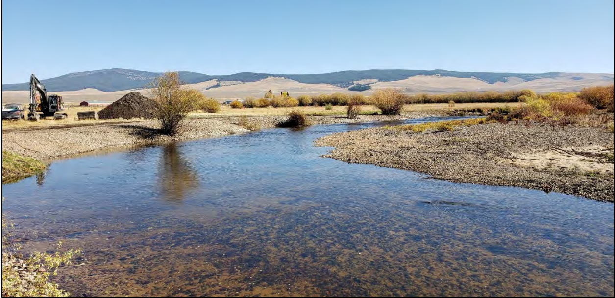
Streambank 1 temporary fix.
