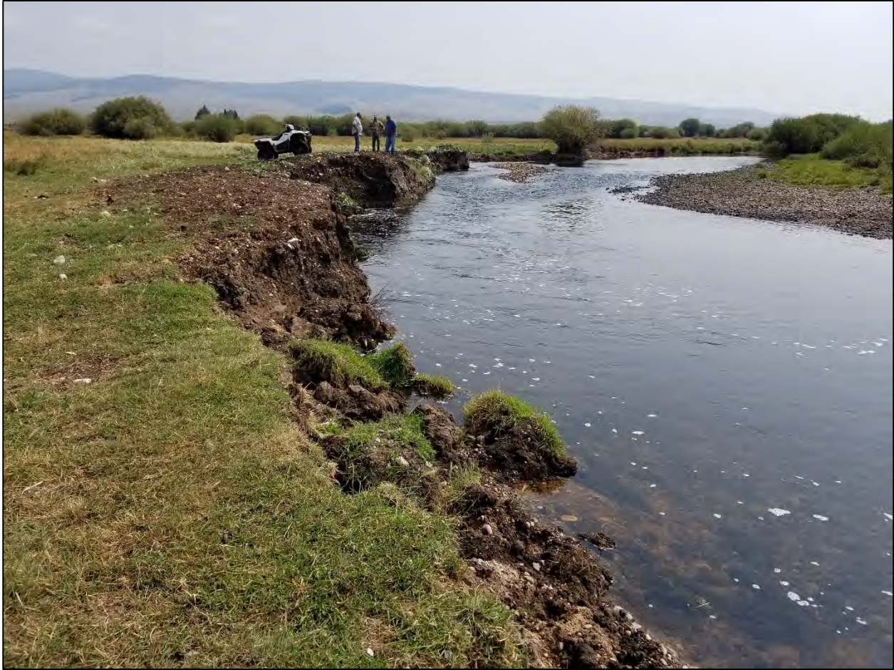
Streambank 1 prior to temporary fix.
